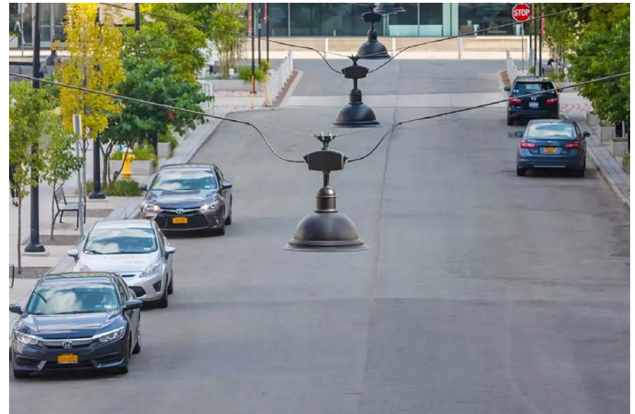
Omega Luminaires with Catenary Mounting over Roadway
